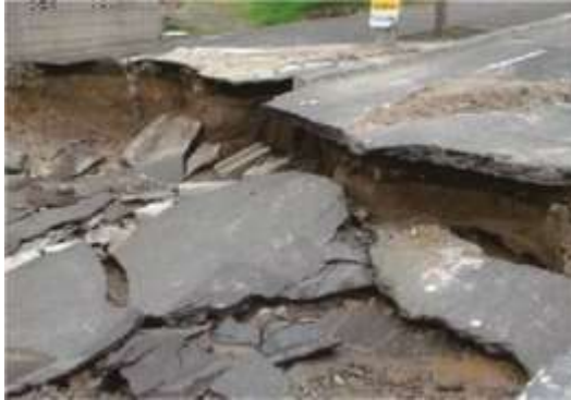
Figure Roads caved in caused by ground subsidence (Hiraoka District, Kiyota District, Sapporo City)
