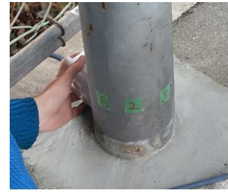
Fig.2. Inspection of corrosion under ground level of sign pole.
