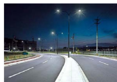
Energy-saving effects with LED lighting. Power consumption reduced by approx. 60% (relative to high-pressure sodium lamps)
