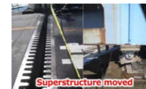
2022 Fukushima Earthquake in March 2022 (Date Bridge, Fukushima Prefecture)
