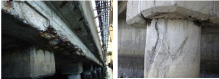
Corrosion of the main steel reinforcement of the reinforced concrete girder
