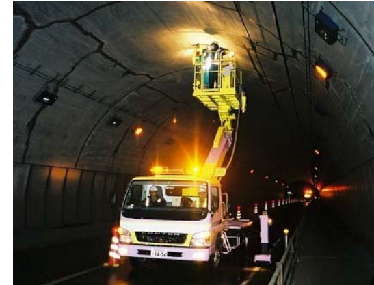
Close-range visual search for cracking
