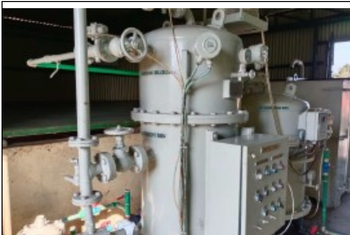
Oily water separation device
