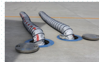
Pits for air-conditioning air
