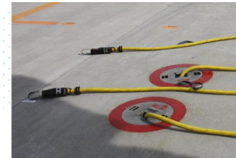
Pits for electric power
