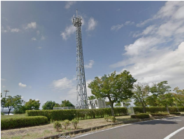
NTT base-station equipment for mobile communications
