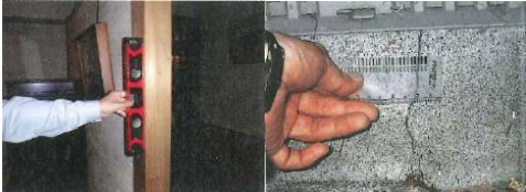
Left: measuring tilting of a post with a level Right: measuring crack width of a foundation with a crack scale
