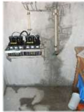
[室内への漏水]
