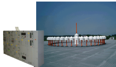
超短波全方向式無線標識施設／距離情報提供装置 VOR/DME:VHF Omnidirectional Radio Range/ Distance Measuring Equipment
