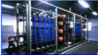
Filter type water processing unit
