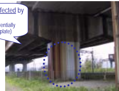
Mid Niigata Prefecture Earthquake (seismic intensity of 7) / Toka-machi, Nagaoka-shi
