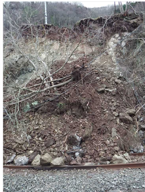
<Status of the collapsed slope >
