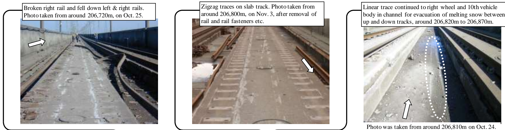
Figure 2. Status of Damages of the Tracks I (4/7)
