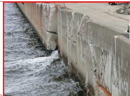
Photo 3 Damage to the Seawall (Excerpt)
