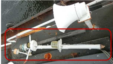
(1) Fractures of the mast, fallen from its original place
