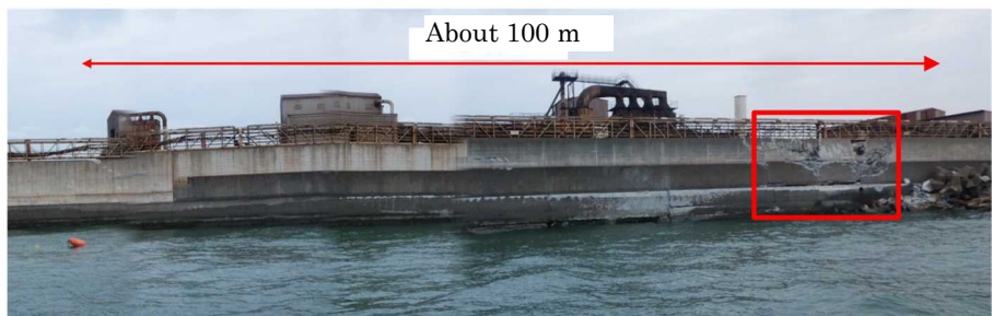
Photograph 3: Situation of damages to the seawall
