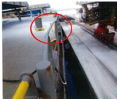
Photo 3: Damage to the handrail
