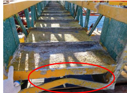
Photo 4: Damage to the gangway
