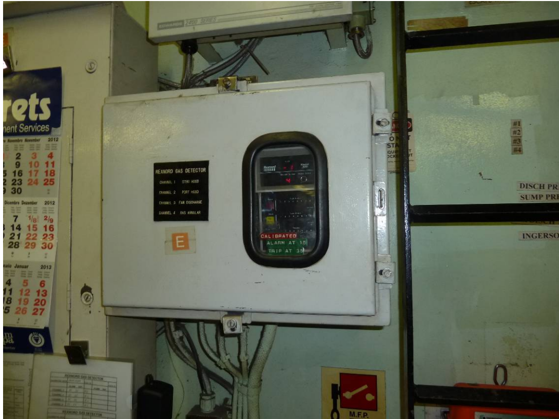
Photo 7: Gas Leakage Detector Monitoring Equipment
