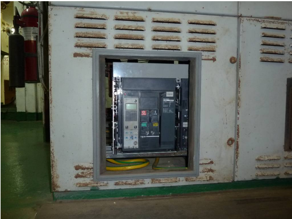
Photo 6: ACB for the Emergency Diesel Generator
