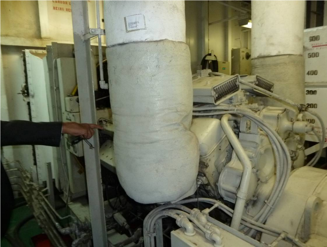
Photo 3: Emergency Diesel Generator (diesel engine)
