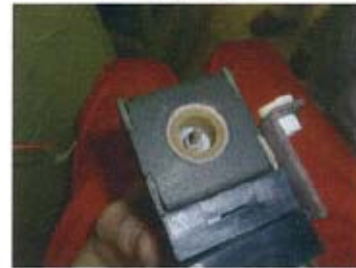
Damage to the solenoid valve for closure operation
