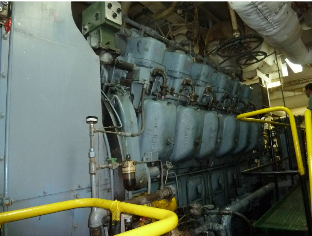
Photo 2: Stand-by Diesel Generator (the port side)
