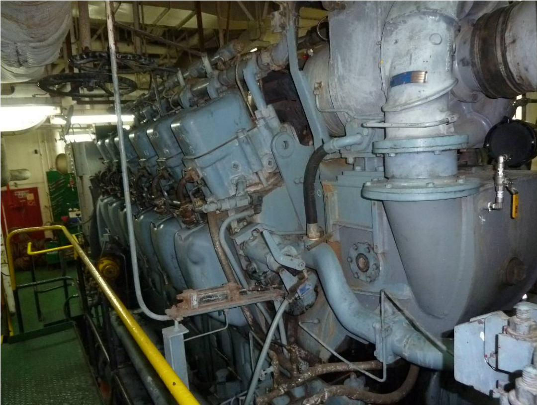
Photo 1: Stand-by Diesel Generator (the port side)
