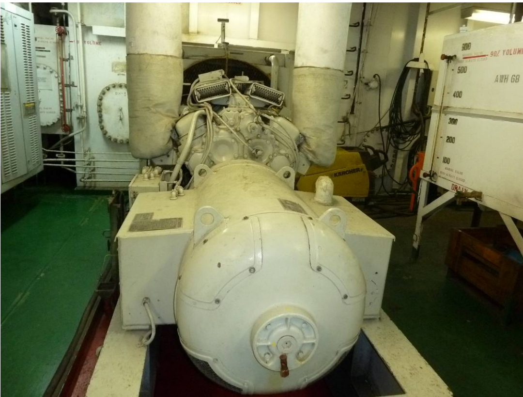
Photo 4: Emergency Diesel Generator (generator)
