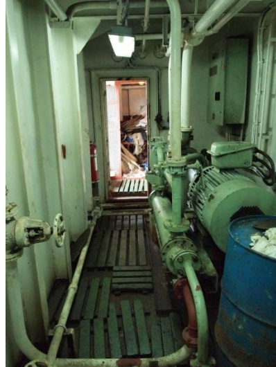
Photo 5: Inside of Pump Room (Seen from the port side)
