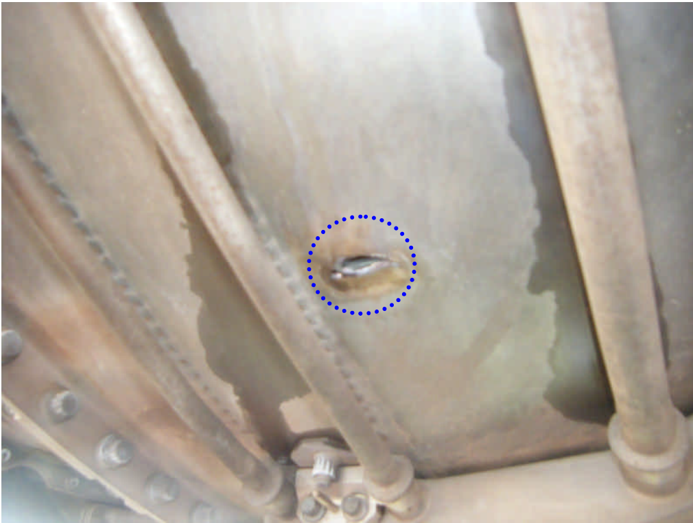
Photo 6 Damaged LPT Casing of No.3 Engine
