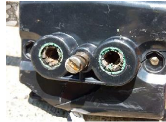
Fig. 2.12.7.3: Damage on J3 Cable Connector
