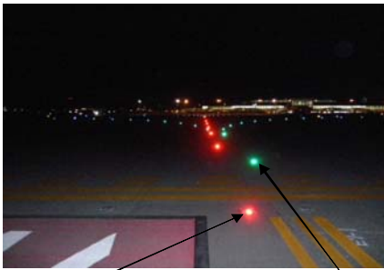
REL Light at the center line of the taxiway
