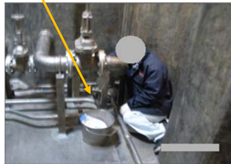
Situation when the chief engineer found 2/O (inside portside No.1 tank)
