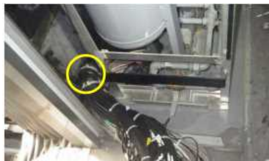
Wired status viewed from aisle side, broken in back side of the circled bundle of cables
