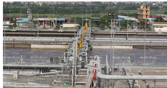
Yen So WWTP, Hanoi
