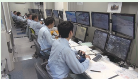
Remote control room
