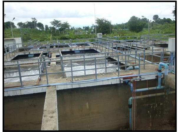
AERATION TANK OF SEWAGE TREATMENT PLANT
