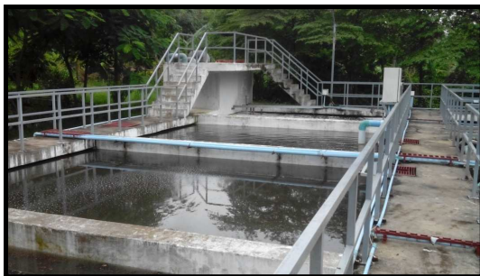
EQUALIZATION TANK FOR SEWAGE COLLECTION
