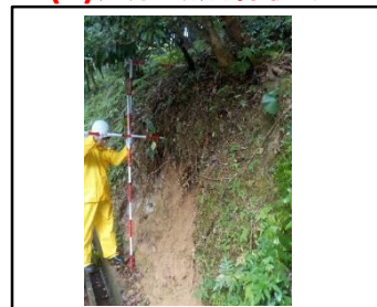
(C)法面崩落状況
