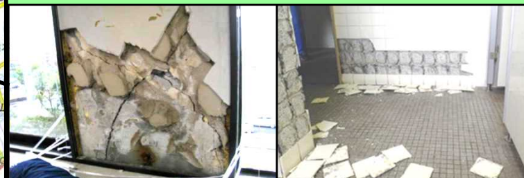
躯体破損、仕上剥落
