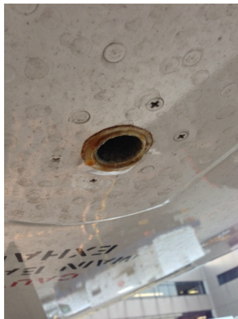
External view of the vent port area
