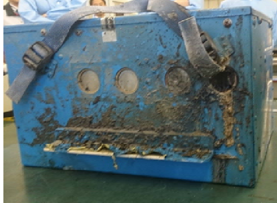
Outside surface of the battery (Only the rupture disk of cell 5, most right, was ruptured).
