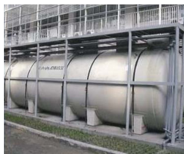
Hospital sewage (Vietnam 50m3/day)
