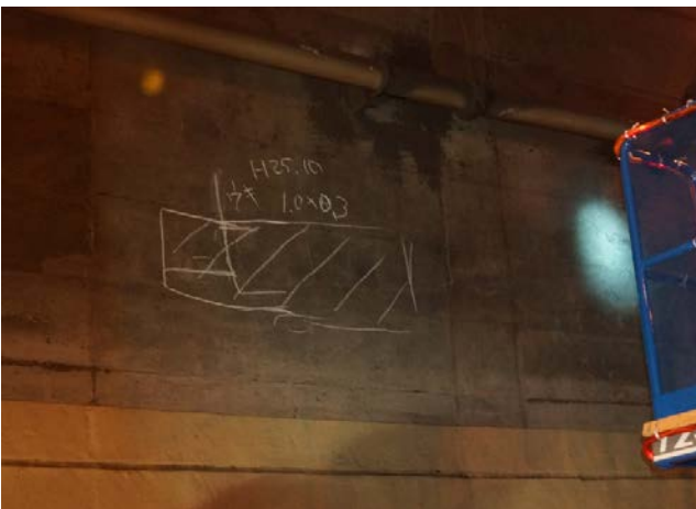
Photo. 4.5 Hammering test in Takashima tunnel. (a) image of high-place work, (b) defective part.
