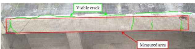
Fig. 4.8 Side view of inspected structure. Green line : position of visible cracks, red line : measured.
