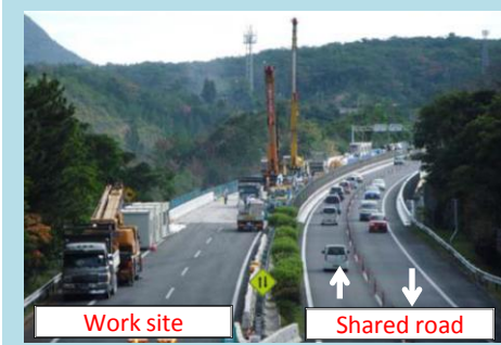
Avoid road closure by having traffic share a road with traffic going in the other direction.
