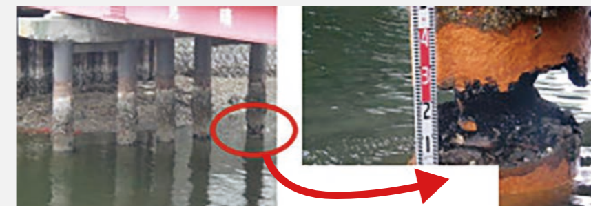
37-year old Miharashi Bridge (on Shinyamashita 8th municipal road) was found damaged.
