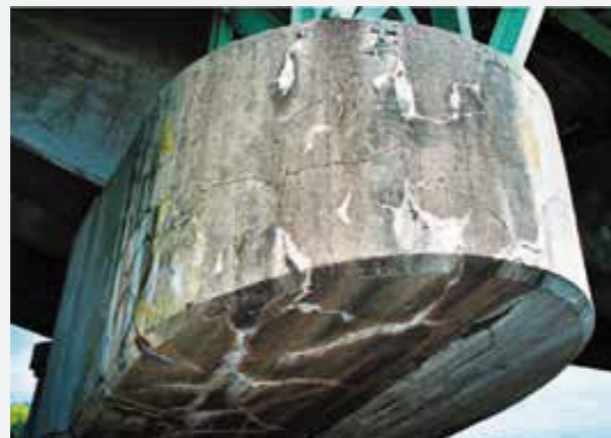
Deterioration due to an alkali aggregate reaction
