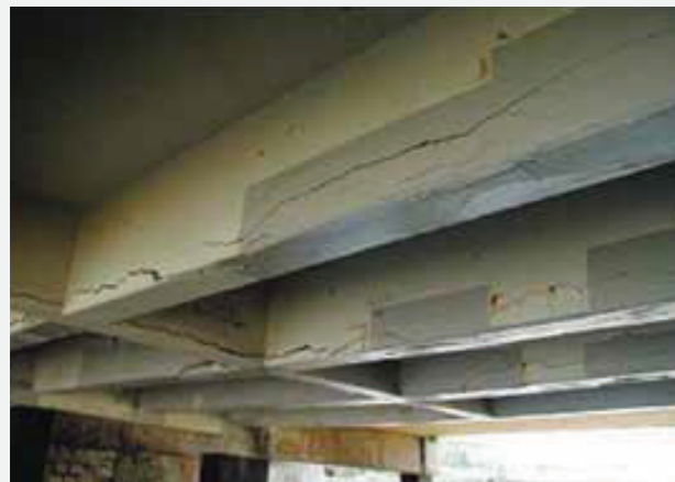
Deterioration due to salt damage
