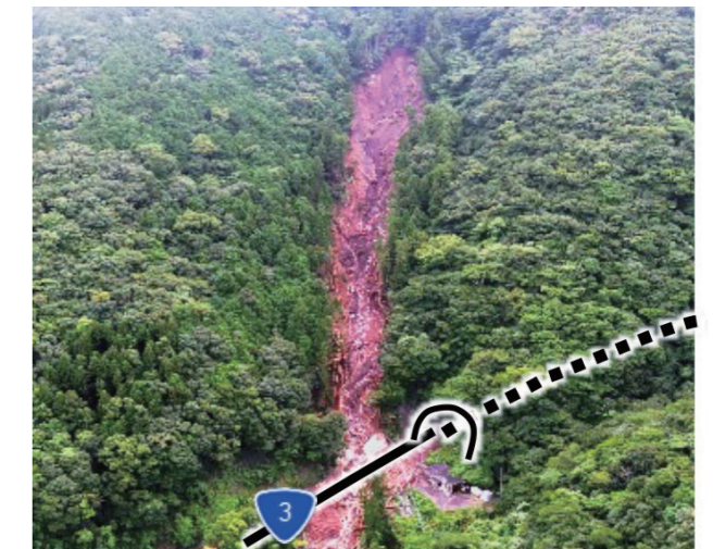
Massive collapse from the top of the slope Heavy rain in July 2020 (National highway 3, Ashikitamachi Kumamoto Prefecture)
