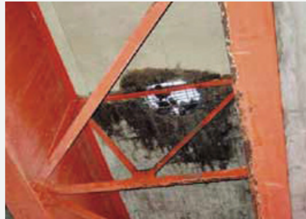
Collapsed slab due to fatigue
