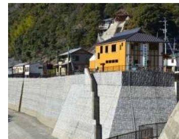
Retaining wall using imitation stone so that it would not affect the landscape
