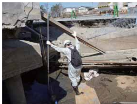
庁舎の被災状況調査 Situation Regarding Damage to Government Buildings and Facilities
